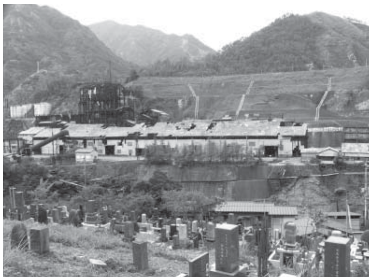
The smelter being demolished, viewed from the Ryuzoji Temple on the other side of the Watarase River (Autumn 2009). Many of the people involved with Ashio are laid to rest in the graveyard at the Ryuzoji Temple. And now, June in 2010, the demolition is almost over.
